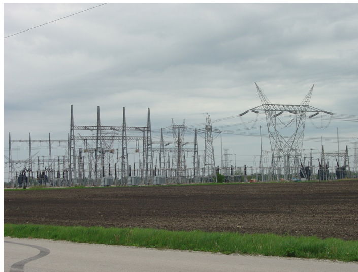
FIGURE 1.6-4 Substation in the Vicinity of Manhattan, IL (Source: Argonne Staff Photo)
