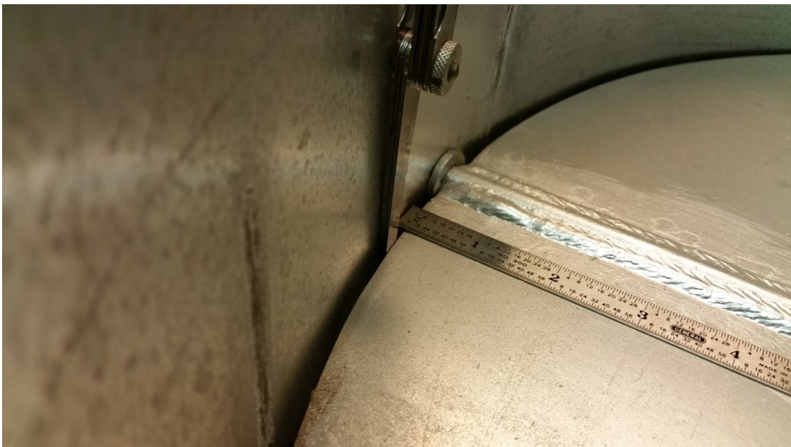
Figure 113: Gap between butterfly valve and inner ductwork. Average gap across entire circumference of 0.125-in
