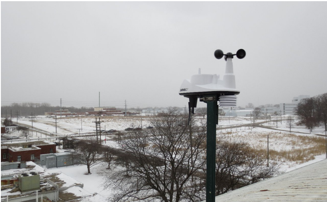
Figure 33: Picture of weather station of Bldg. 308 roof top
