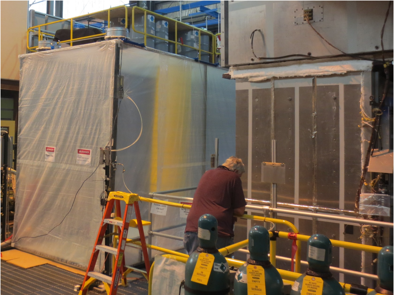
Figure 101: Argon enclosure constructed above downcomer inlet
