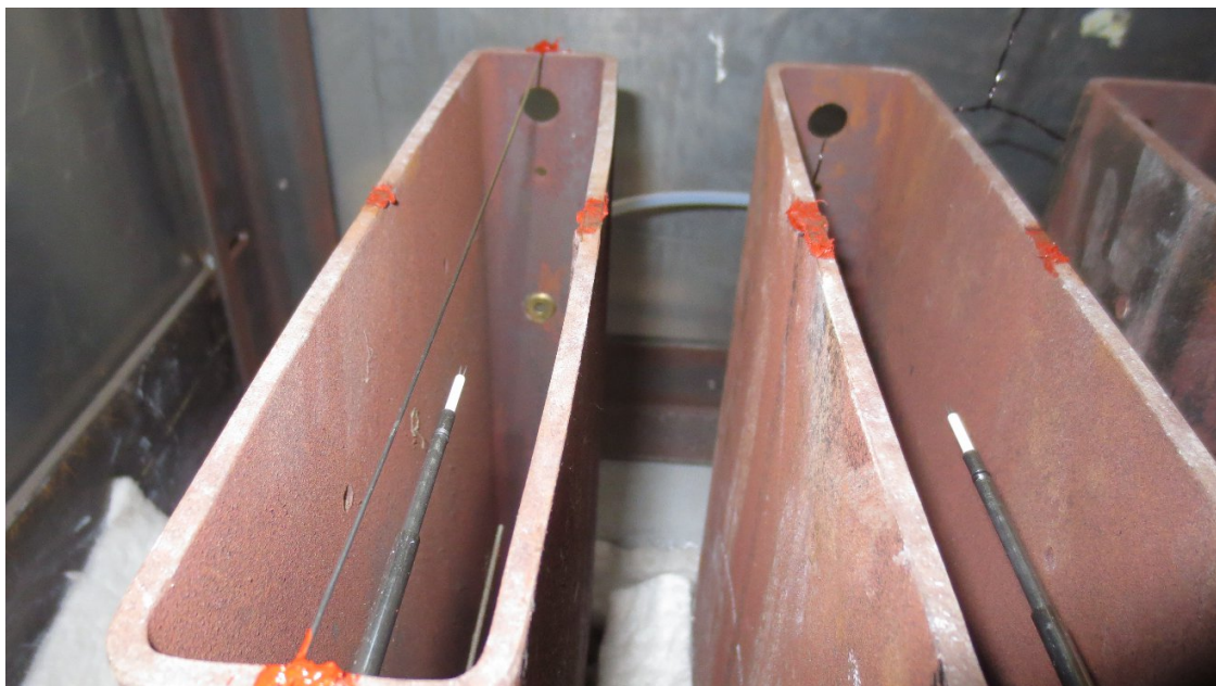
Figure 50: New LUNA fiber sensors installed across 10-inch width of one riser duct (outlet)
