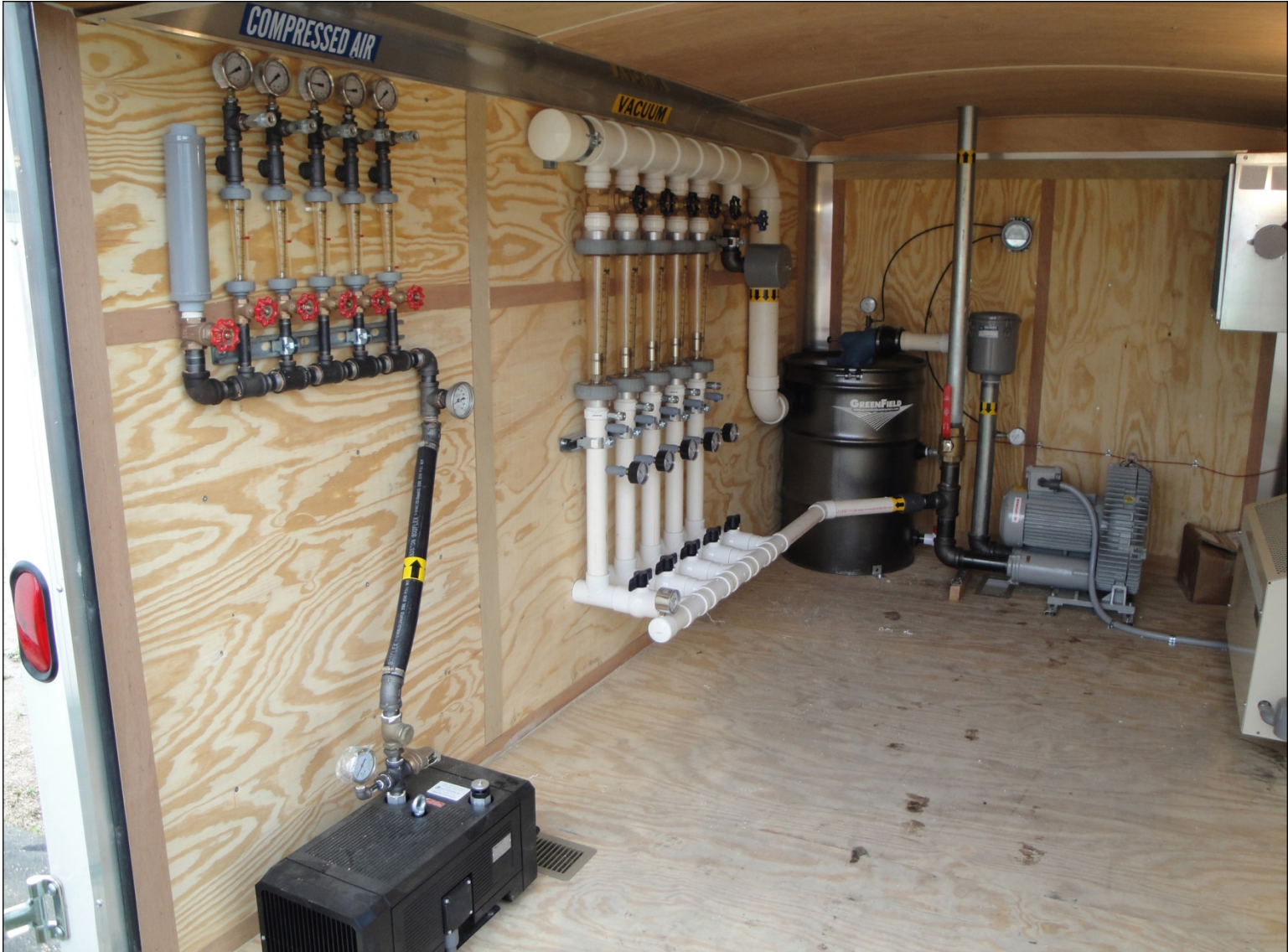
FIGURE 2.3 The compressed air and vacuum lines in the SVE/AS equipment trailer.
