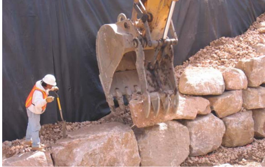
Figure 1-1: Example dry-stack rockeries built as retaining structures. Photo source: CFL staff from the “Beaver to Junction Project” in south-western Utah; project designed by CH2MHill
