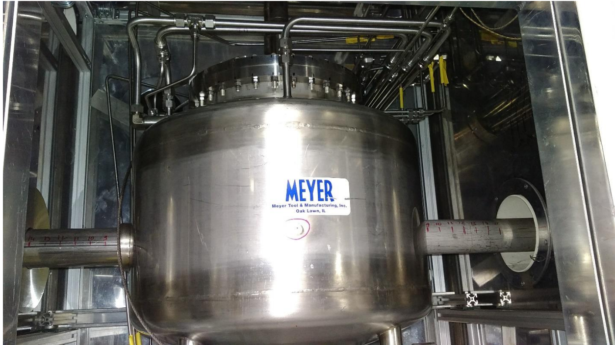
FIGURE 2.1.3.3 Target solution vessel and depleted-uranium target installed inside the shielded cell
