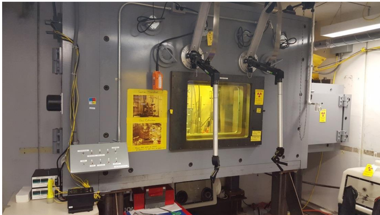
FIGURE 2.4.1.1.1 The D-024 Hot Cell, where final purification of ^{99}\text{Mo} is performed
