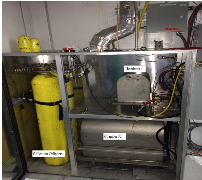
FIGURE 2.2.2.7 Photograph of the gas collection system inside the enclosure
