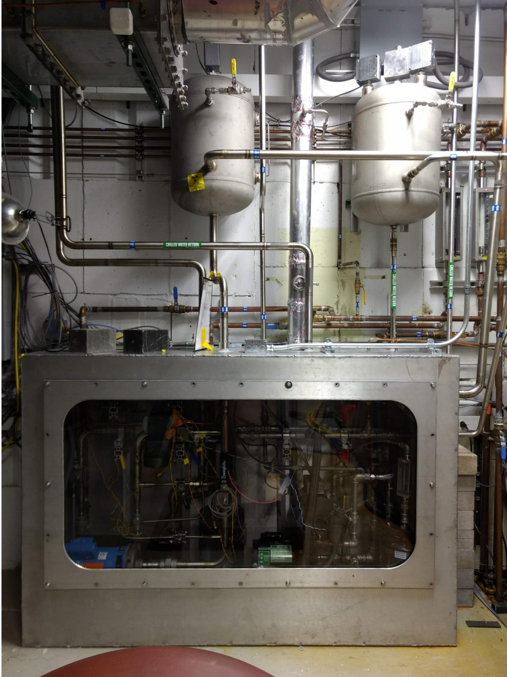
FIGURE 2.1.2.4 Cooling system for target solution vessel and DU target
