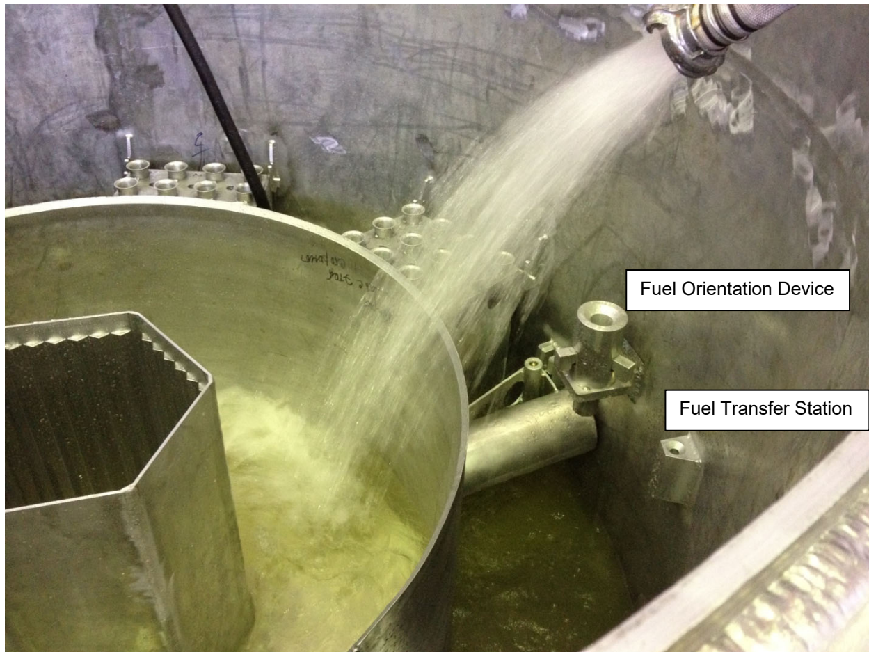
Figure III.7.3. Interior of the SCA tank is shown being filled with water during manufacturing testing. Two fuel racks (upper left and center), one neutron beamline channel can (center right), the fuel orientation device, and the fuel transfer station are visible in this photo. The graphite reflector ring fits in the space being filled with water, between the hexagonal part of the SCA and the circular aluminum wall; about half of the space is shown in this photo.
