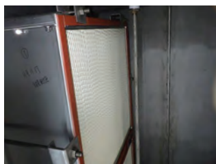
Inside of the Unit 3 SGTS filter train (HEPA filter)
