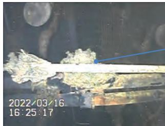
Deposits suspended on piping above water level
