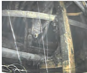
Thread-like deposits above water level
