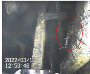
Thread-like deposits above water level
