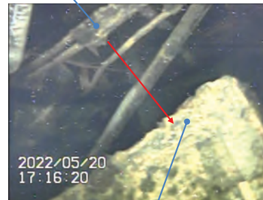
Deposits suspended on structures in water (shielding of equipment drain sump pump)
