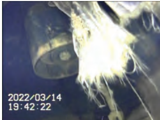
Damaged lead wool blanket with exposed fibers
