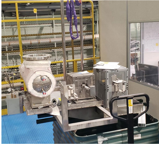
Figure 58: AHX installed on the secondary component support platform along with flowmeter and pump. The heat exchanger, flowmeter and pump were secured to the platform and hoisted as one unit to mount to the platform to the vertical support column. The components were then unbolted to allow for thermal expansion as required by ASME B31.3 piping analysis
