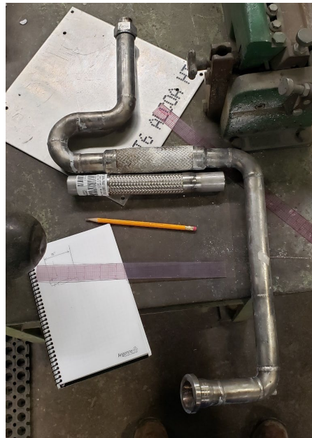
Figure 36: Swollen, damaged expansion joint shown as welded into the piping. New expansion joint that was welded in shown immediately below.
