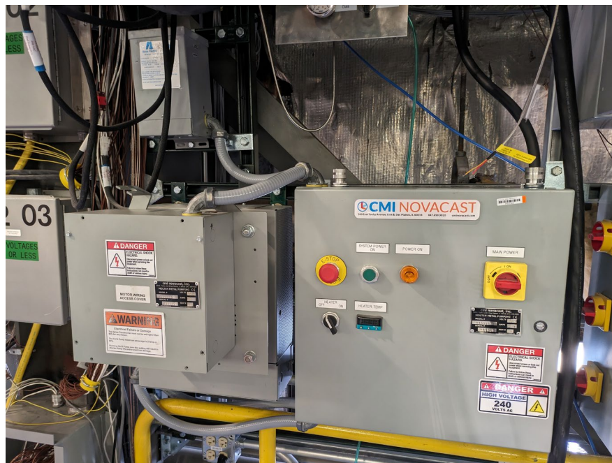
Figure 61: Three electrical cabinets installed for AC conduction pump.
