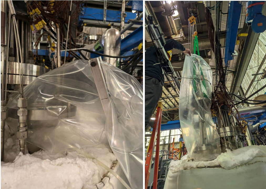
Figure 55: Photos showing the installation of the IHX with the use of the overhead crane and a custom glovebag. On the left the glovebag is being cinched shut with a custom clamp as the glovebag is being inerted with argon. On the right the assembly is being inserted into THETA.
