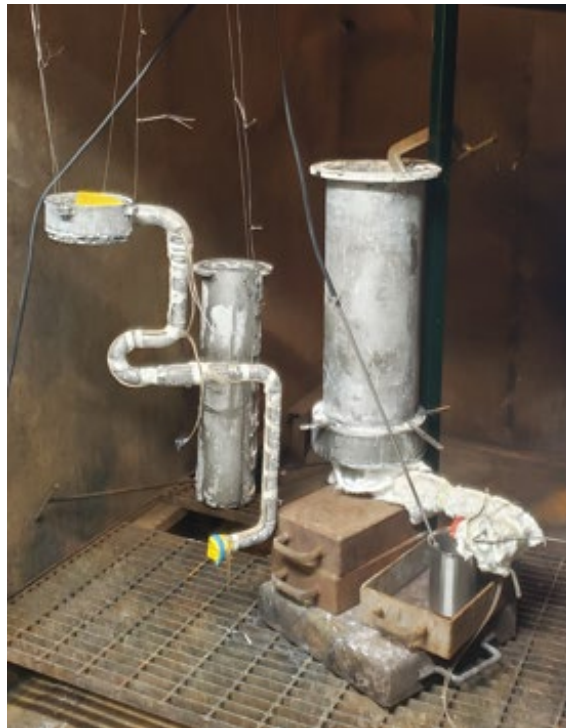
Figure 34: Photo showing the THETA cold pool components with trace heaters and insulation installed. Components oriented to facilitate drainage. Catch pan and argon gas line to inert the pan shown under core barrel piping, prepared for sodium melting.
