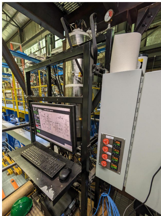
Figure 19: Photo of the carbonation system showing the control computer, process heater controllers, and CO 2 sparging tank.
