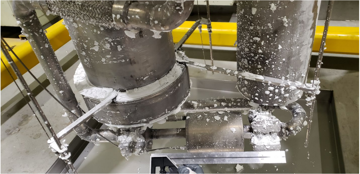
Figure 22: Photo showing sodium (bi) carbonate residue on the lower cold pool ponents.
