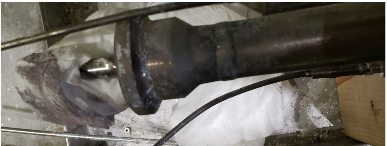
Figure 33: Drill bits were used to remove bulk sodium from the flowmeter, top. The drill bits were treated in the burn stall to remove bulk sodium from the flutes, middle. Dry lint free wipes were then used to remove loose surface sodium on the inner walls of the flowmeter, followed by lint free wipes with ethanol, then ethanol diluted with deionized water, and finally deionized water, bottom.
