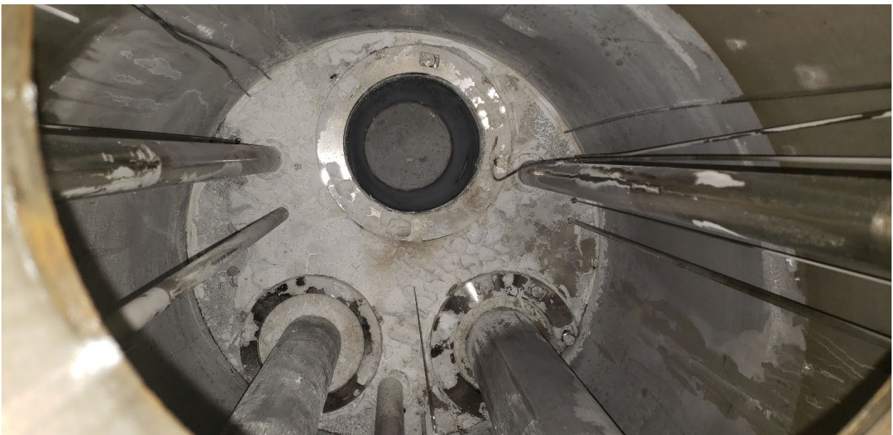
Figure 25: Photo showing the inside of the THETA hot pool inner vessel with the core immersion heater removed. The carbonation process reacted the sodium in this large cavity quite well. The bi(carbonate) was mechanically scraped and a dedicated vacuum was used to remove the biproduct into a plastic bag for sodium decontamination. Small pockets of pure sodium remained under the carbonation product which were cleaned with ethanol then deionized water.
