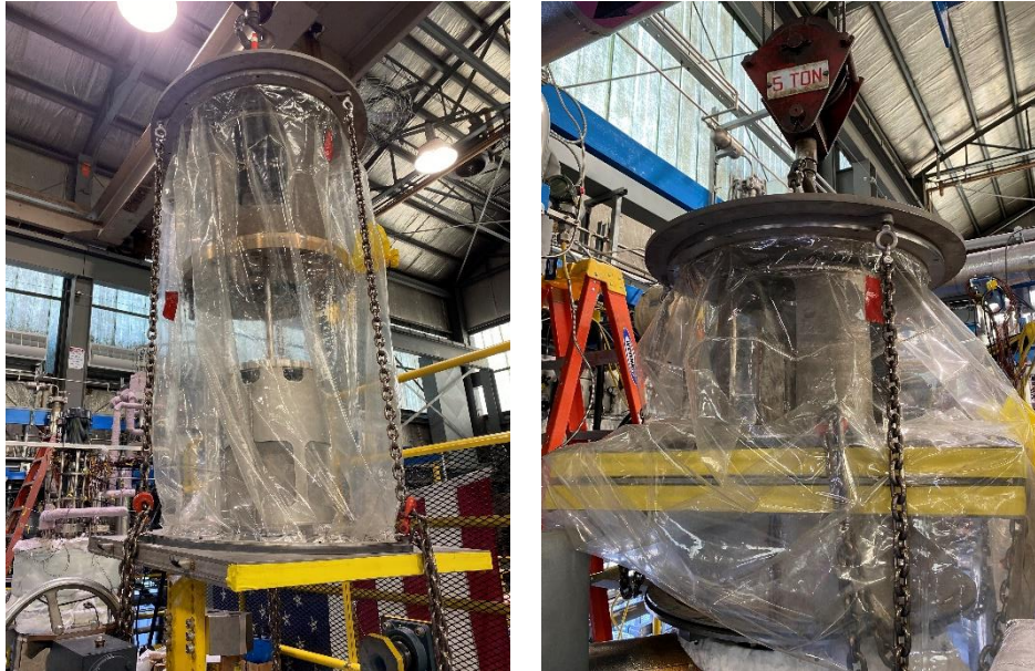
Figure 8 – Assembled STB being lifted from the assembly test stand with the flexicask system (left). The STB installation in vessel 1 using the flexicask system (right).
