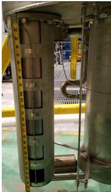
Figure 84: Phot showing IHX outlet thermocouple junction locations
